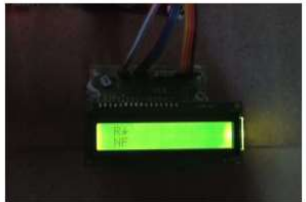
Fig. 7 No Fault Indication
