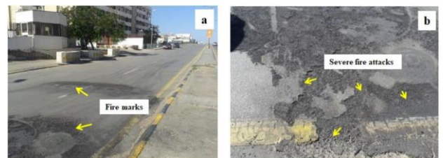
Figure 1: a) A general view of the burned road; b) A369 close view of the damaged location
