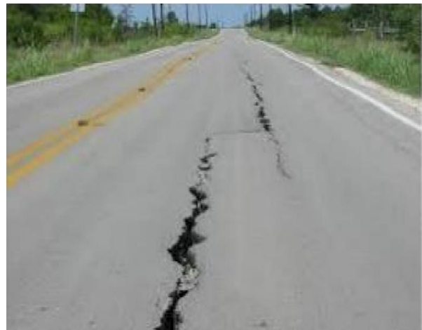
Fig 3. Plate 2.Z Longitudinal cracks in Bitumen Road.
