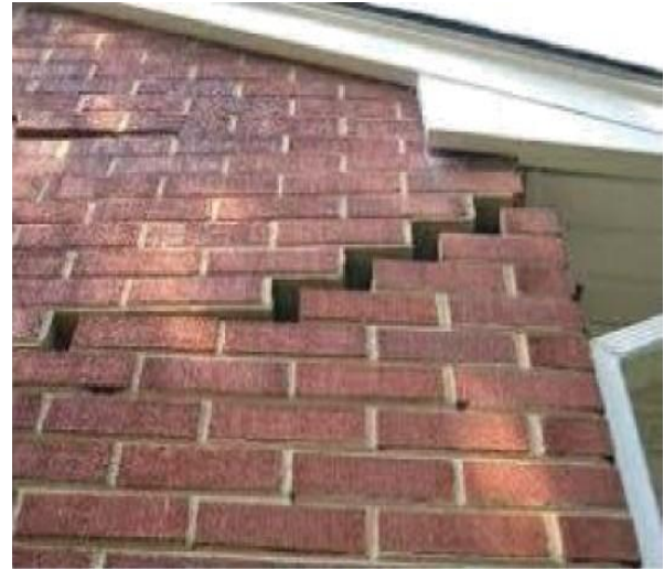
Fig 2. Plate 2.2 Diagonal Cracks due to differential Heave.
