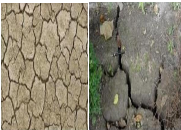
Fig 1. Plate 2.1 Cracks due to Skrinkage of Soil.
