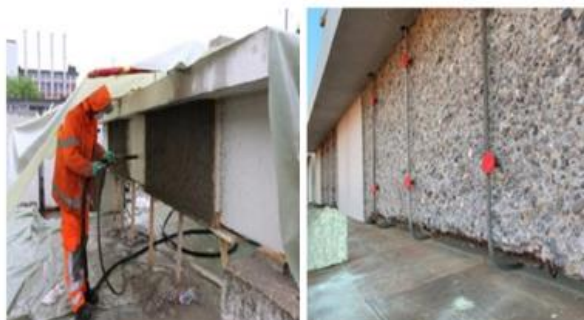
Fig 11. Installed memory-steel stirrups on one of the test beams and application of spray mortar to one of the test beams [40].
