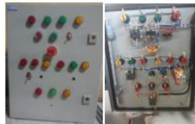
Fig.7. Motor Controller Panel (Figure shown the Control panel and Wiring Connection.
