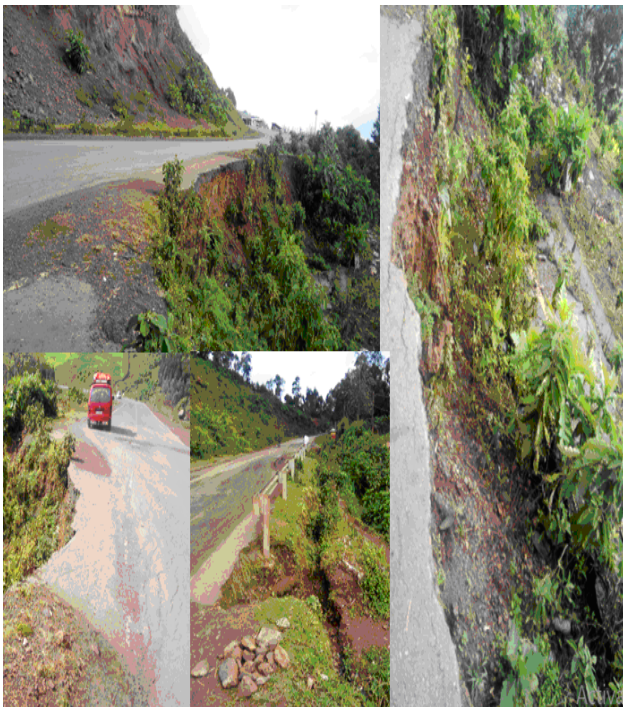
Figure 1: Photograph of the landslide in the Gedo area
