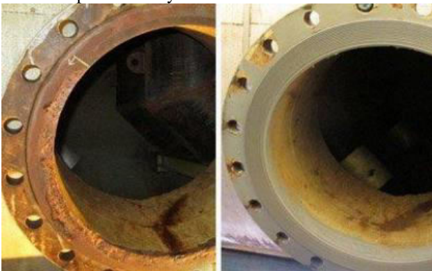
Fig.3. Corroded Pipe and Sprayed with Cold Spray Pipe (Science Direct).
