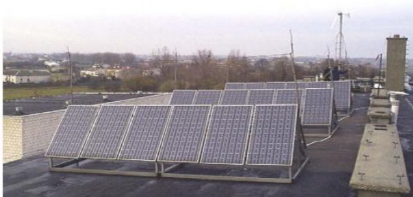
Fig. 3. View of solar panels and wind turbine of the hybrid power plant.
