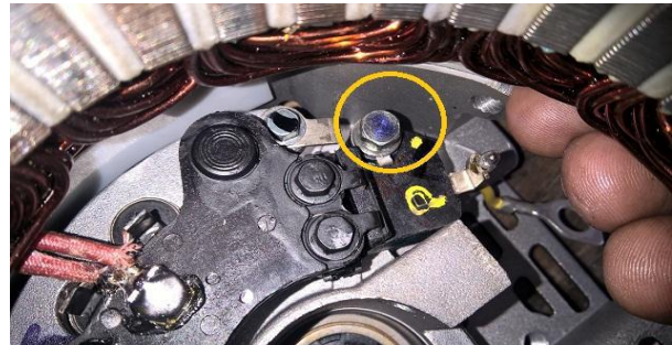
Fig 4 Regulator fixing screw with SRE bracket found in loosened and not tightened fully.
