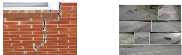
Fig.1 Cause of Damage on Structures
