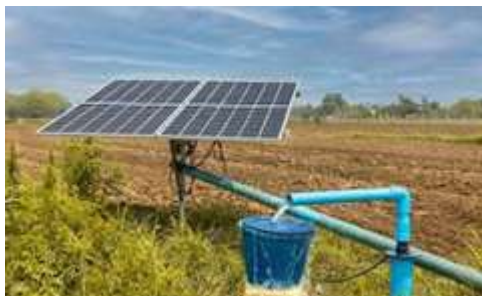
Figure 12 Solar water pump
